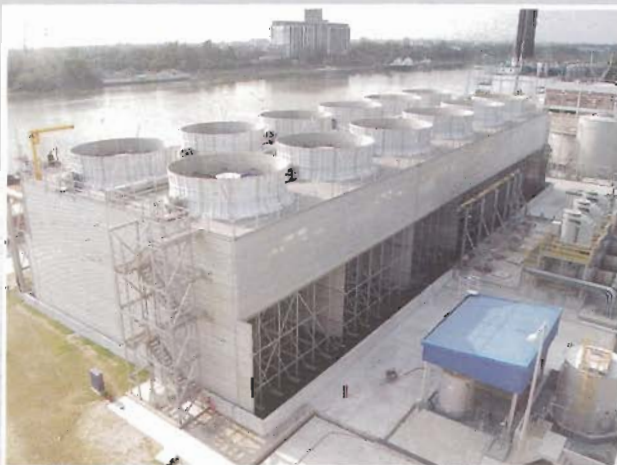
Cooling Tower for Haripur 412 MW CCPPP
