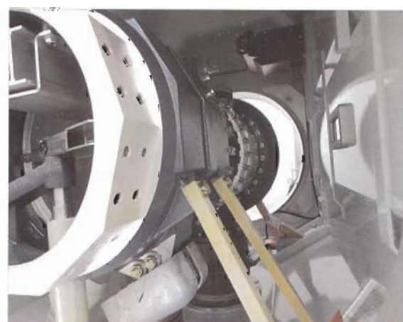
Generator Circuit Breaker
