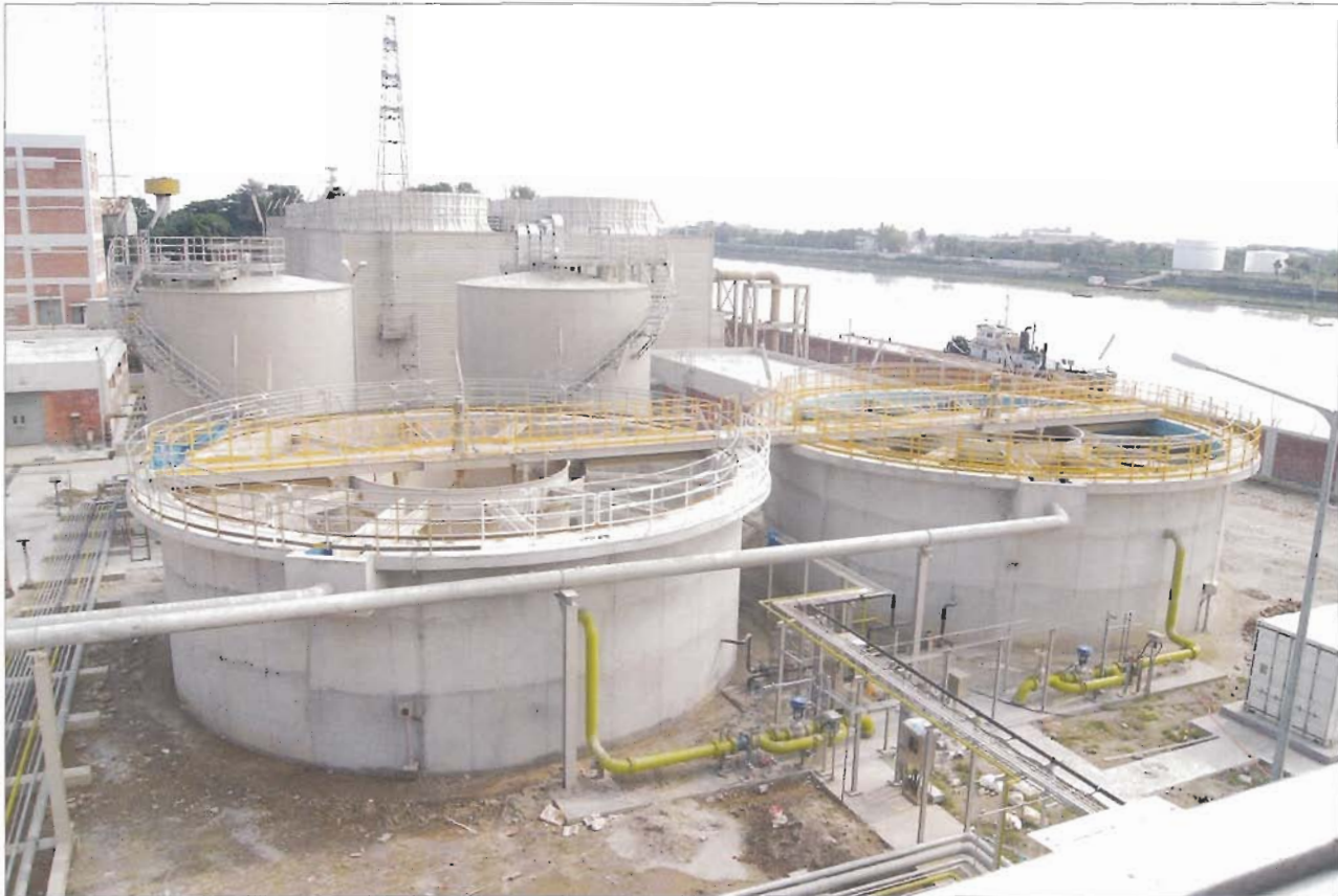
Water Treatment Plant of Haripur 412 MW CCPPP
