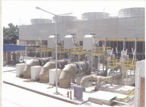
Cooling Tower (Haripur 412 MW CCPPP)
