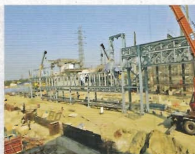
Siddhirganj 335 MW CCPPP
